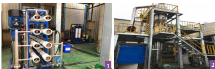
1. CFRO membrane concentration system 2. MVR wastewater forced circulation evaporator
