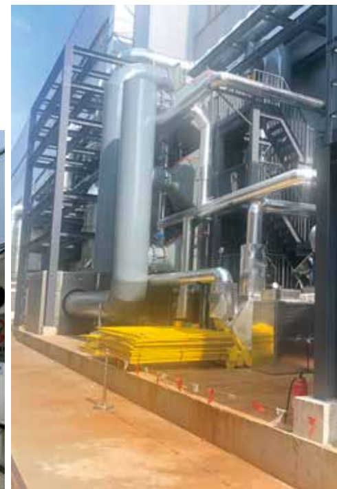
Treatment facilities of spray booth after renovation
